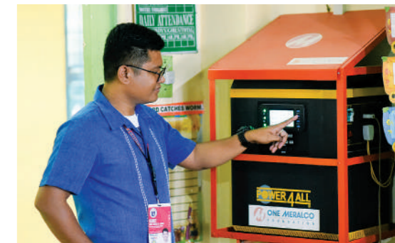
Abing checks the solar equipment installed by the Foundation. OMF trains teachers to conduct basic troubleshooting and maintenance after installation.
