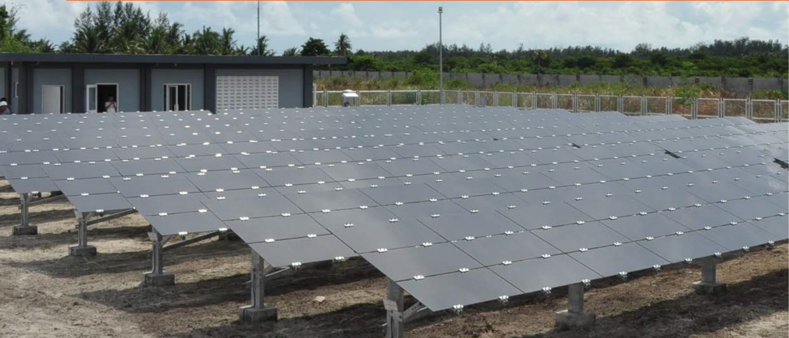
↑ An array of solar panels installed by Meralco in Cagbalete Island, Quezon now provides sustainable electricity to the island's residents.
